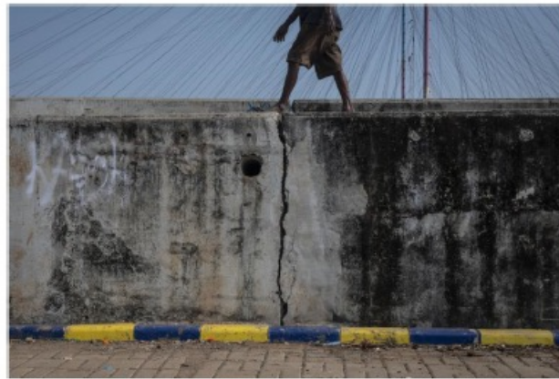
A person walks on a cracked wall on May 7, 2024, in Kalibaru, Cirebon, North Jakarta. Residents of the area fear that the wall, which was built to protect the area from waves and tides, could collapse at any time. (Jakarta Post by Alfar)
